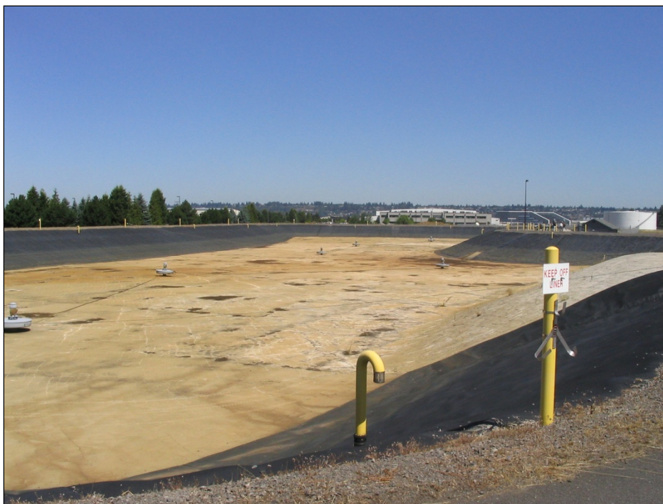
Figure 7-5. Aerated Pond Installation at Portland Airport
