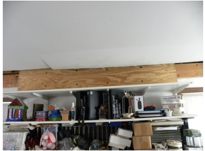
Photo 7: "make shift" supports holding floor
