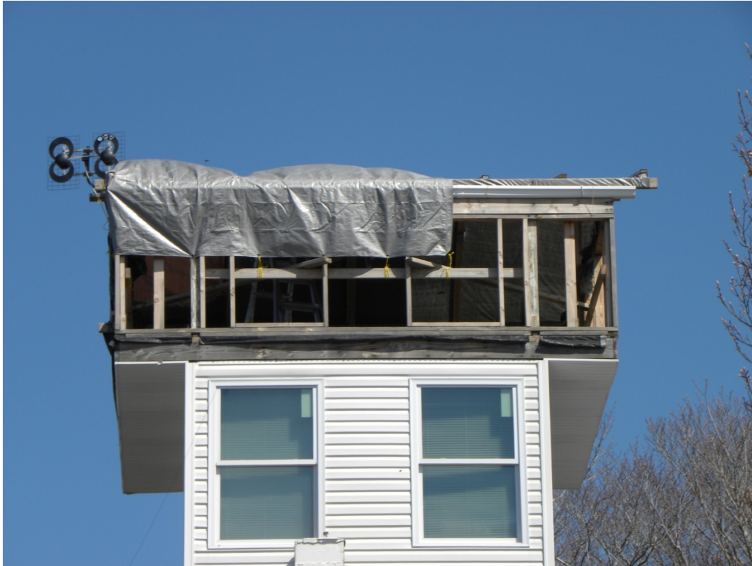
Photo 25: Unfinished, exposed and water damaged fourth floor. Framing is not in compliance with NYS Building code. Note lack of headers over window openings and inadequate framing.
