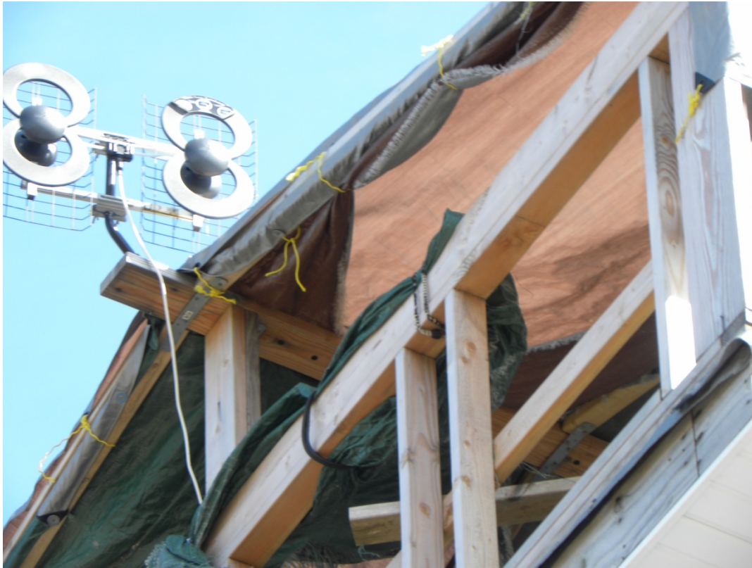
Photo 26: Unfinished, exposed and water damaged fourth floor.
