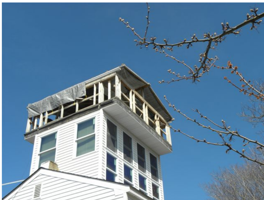
Photo 2: nonconforming third and fourth story
