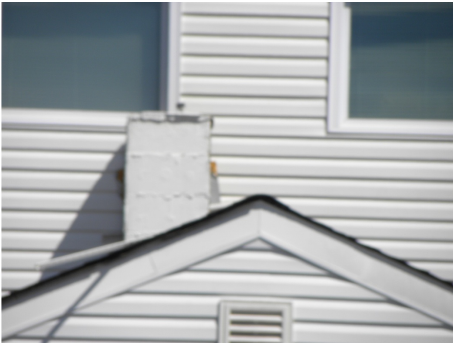
Photo 27: Serious safety hazard due to chimney terminating adjacent to flammable vinyl Siding and below window. Chimney must terminate 3 feet above tallest point and 3 feet Away from any windows.
