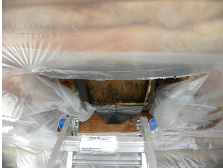
Photo 23: Photo of hatch leading up to fourth story showing water damaged lumber and plastic intended to slow infiltration of rain water.
