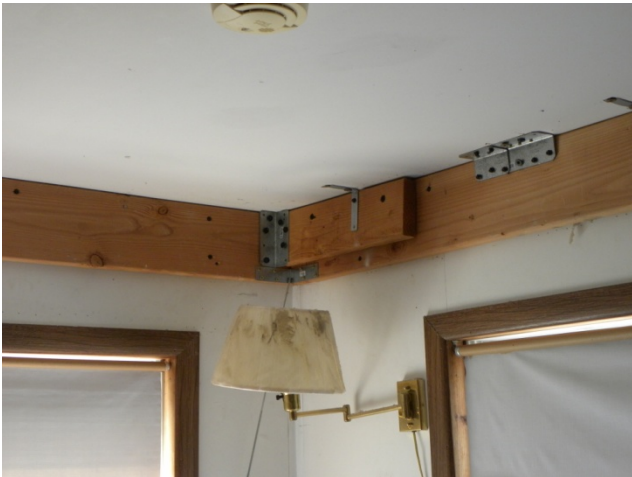
Photo 8: more non-compliant supports and brackets supporting third and fourth floors.
