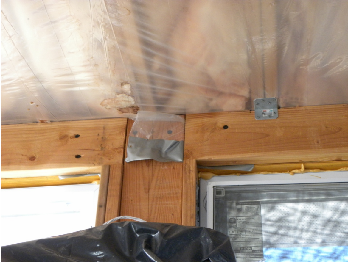
Photo 20 showing insufficient non-code compliant single "jack studs" supporting window header
