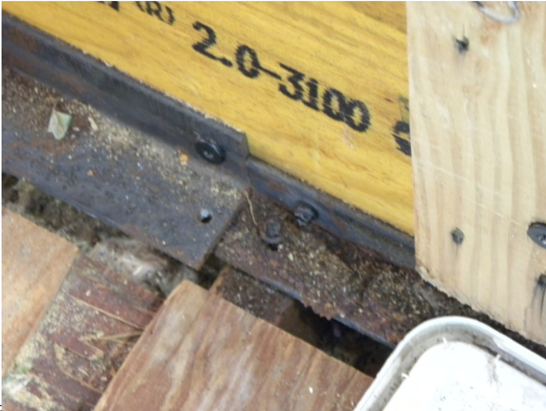
Photo 23: Inadequate and misapplied angle iron screwed to walls.
