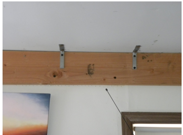
Photo 9: closeup of flimsy shelf brackets and header screwed to Through sheetrock wall and into vertical wall studs.
