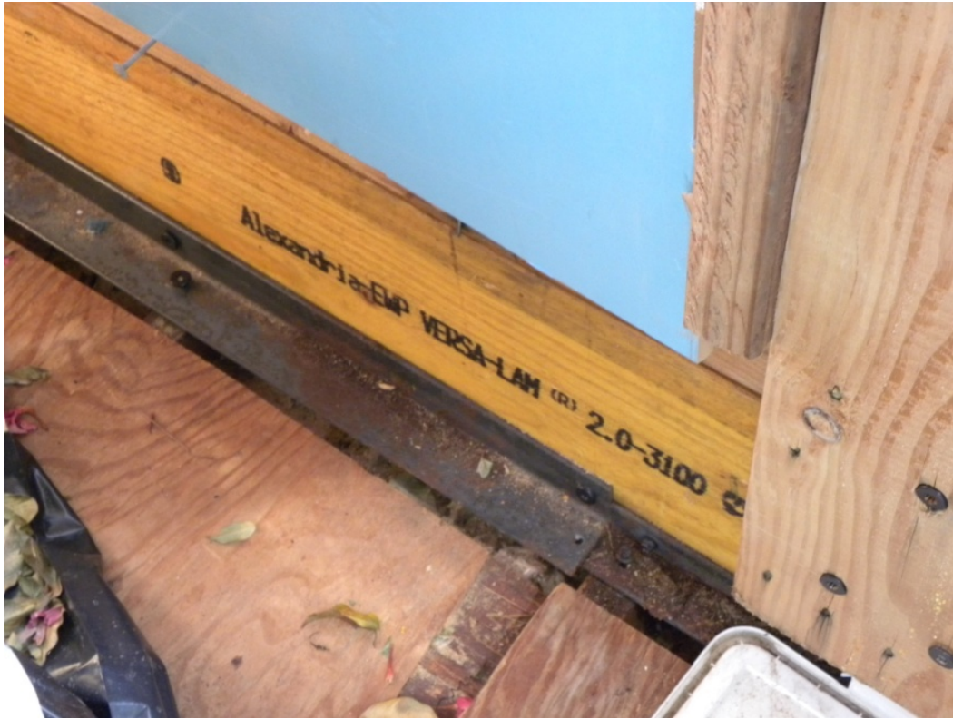
Photo 22: view of inappropriate hardware store angle iron along base of wall. This angle iron is not providing any structural strength to the building addition.
