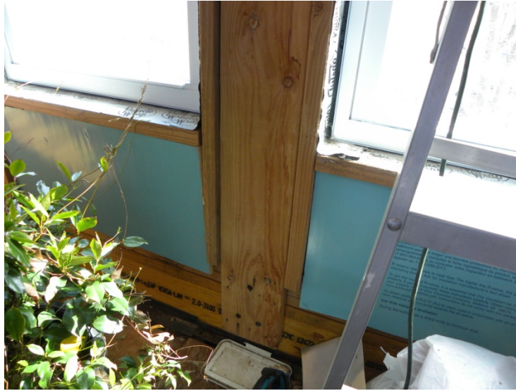
Photo 22: Notice single 2" x 4" wood studs that support header over the window. Studs should be double (2) studs and MUST reach the supporting member below.
