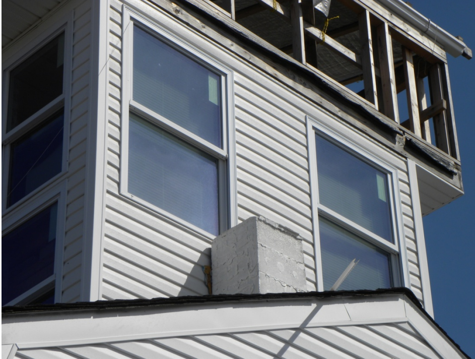
Photo 28: Serious safety hazard due to chimney terminating adjacent to flammable vinyl Siding and below window. Chimney must terminate 3 feet above tallest point and 3 feet Away from any windows.
