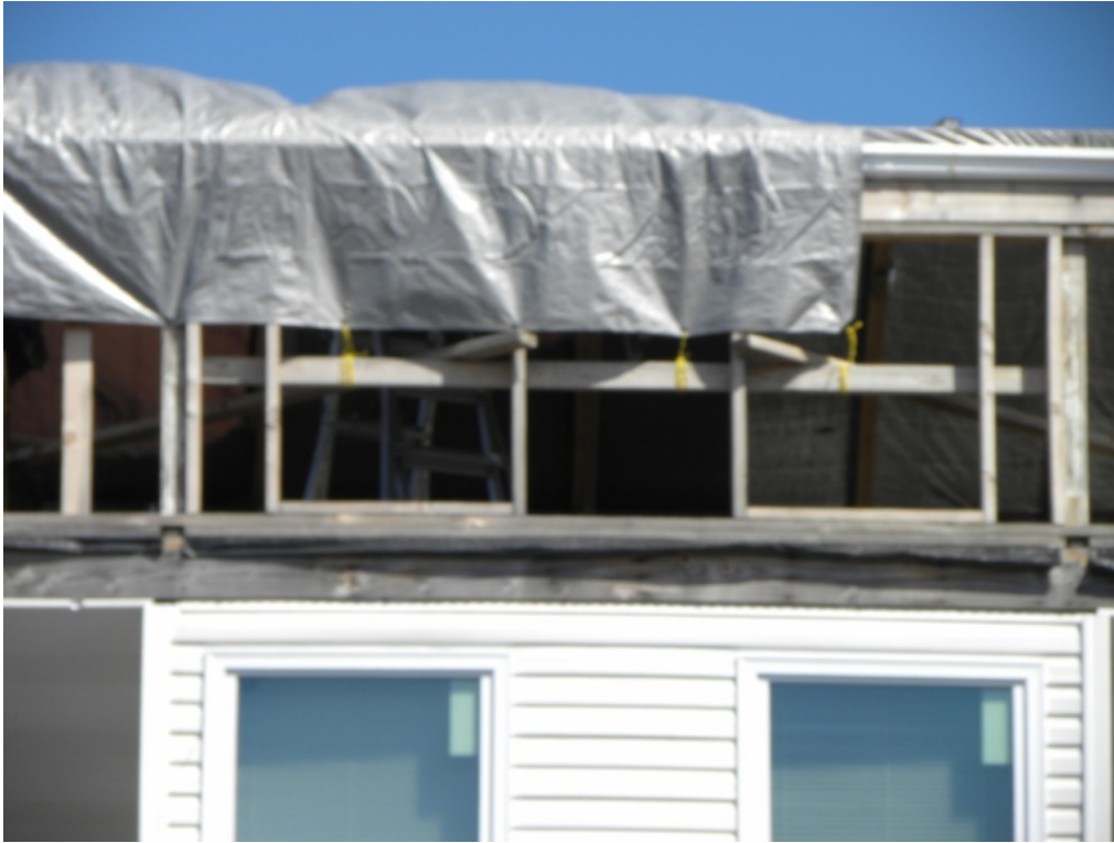
Photo 24: Unfinished, exposed and water damaged fourth floor. Framing is not in compliance with NYS Building code. Note lack of headers over window openings and inadequate framing.
