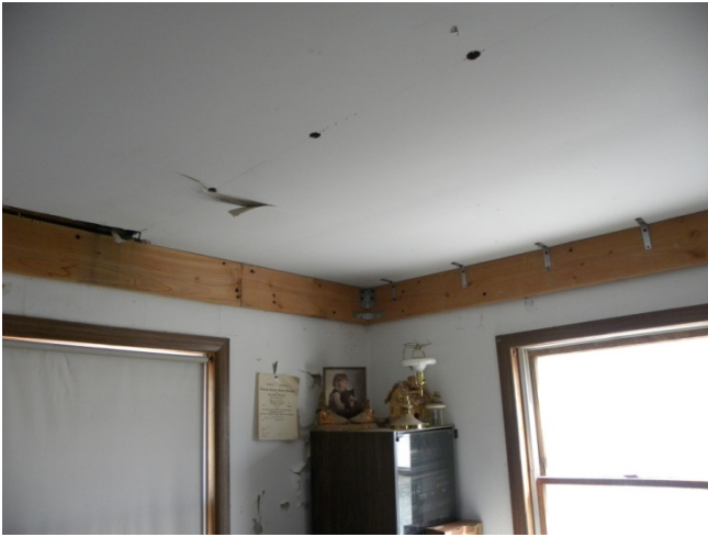
Photo 6: second floor ceiling showing wood headers and above Flimsy metal hardware store shelf brackets.
